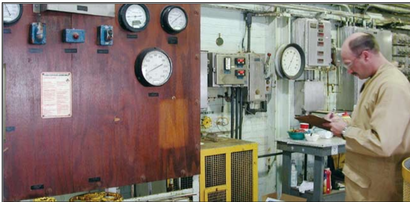
The control room for the Ammonia Oxidation Plant where dilute nitric acid is produced and is later concentrated in another part of the plant.
