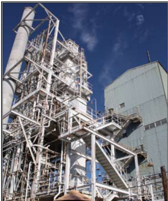
Modernizing the acid plant at Radford is key to its ability to ensure production of nitrocellulose.
